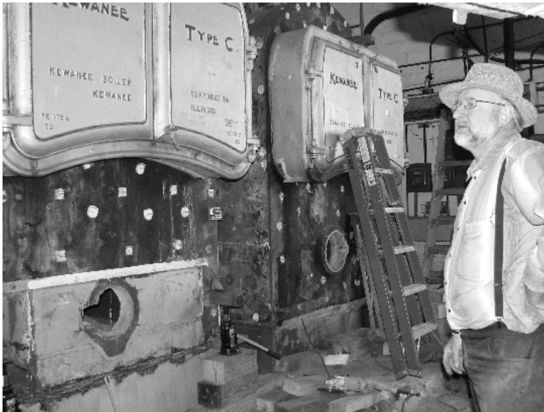
Joe Waldner, the manager of the Mayfield Colony, checks progress on the removal of the boilers with two left to go. The three boilers used to deliver steam to all of Westmar's campus. (Photo courtesy of the Le Mars Daily Sentinel.)
